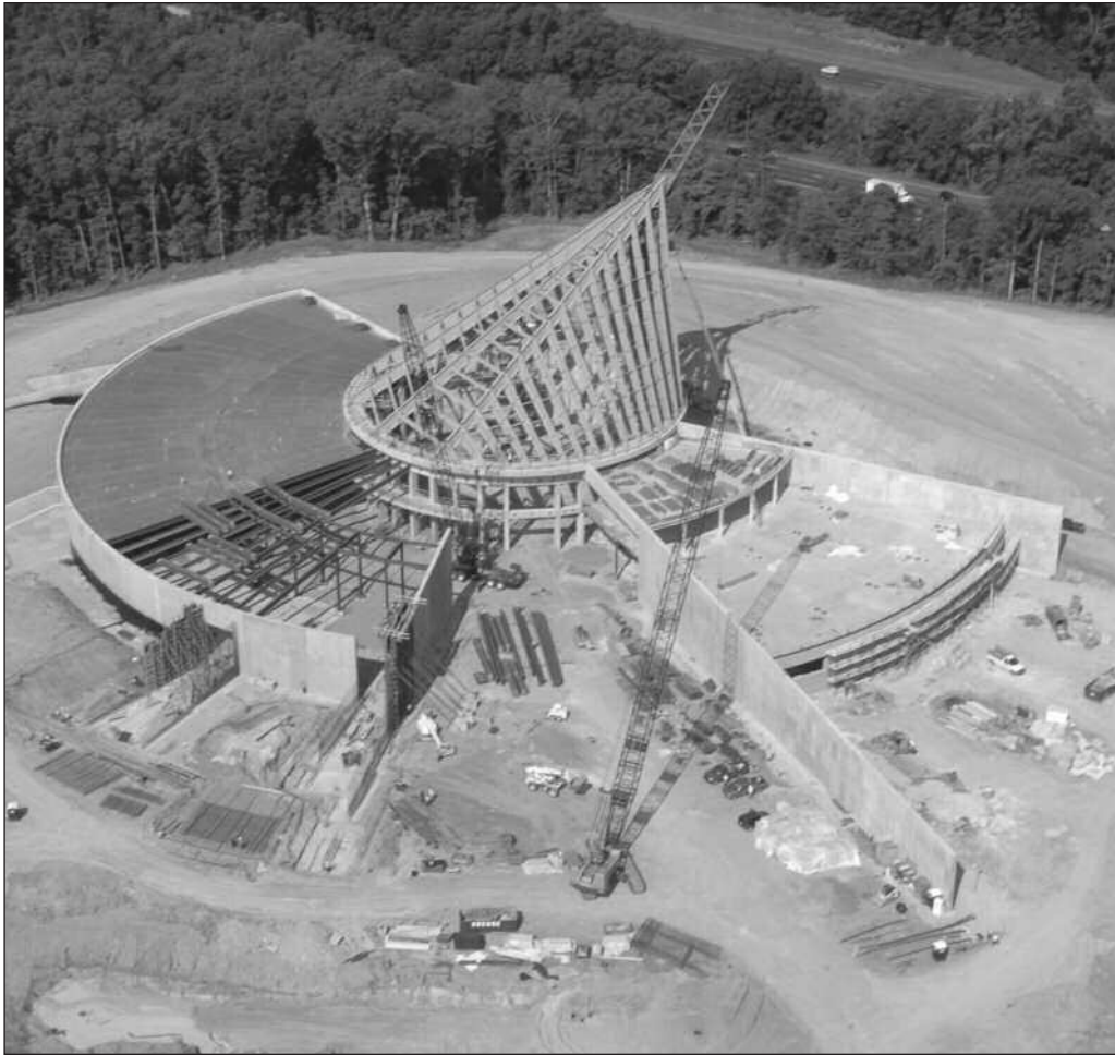
This recent photograph shows the “main mast” and canopy of the National Museum under construction. Worksites vehicles provide a sense of the large scale of the new building.
